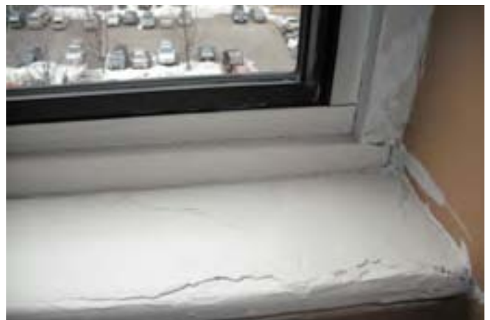
WATER-DAMAGED WINDOW SILL RECORDED IN MCI SURVEY
