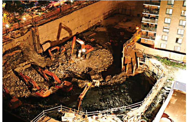
Retaining wall collapse at 784 Columbus Ave. Photo by Nina Berman July 25, 2007
