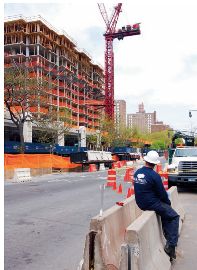
The Department of Buildings found potential problems with parking spaces and curb cuts at this construction project at Park West Village.
